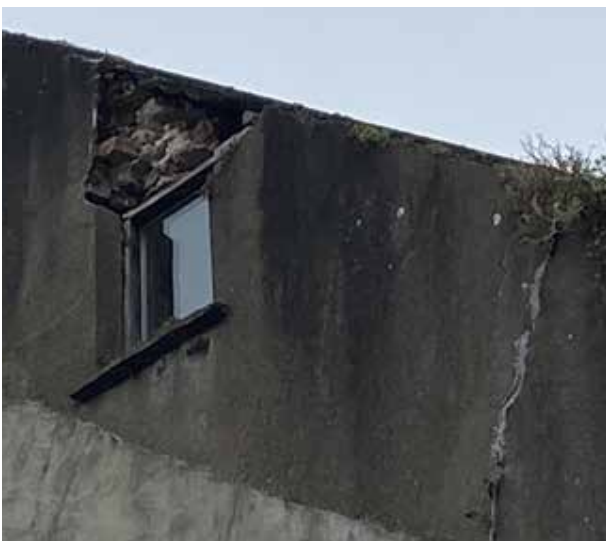
Figure 63 - Poor maintenance, Quay Street
