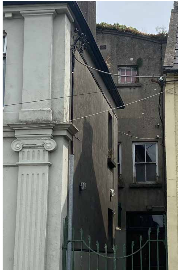
Figure 92 - Poor maintenance evident to structure to rear of YMCA, John Street
