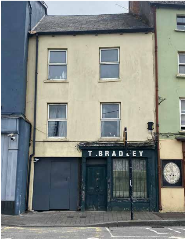
Figure 89 - Subsidence evident, The Quay
