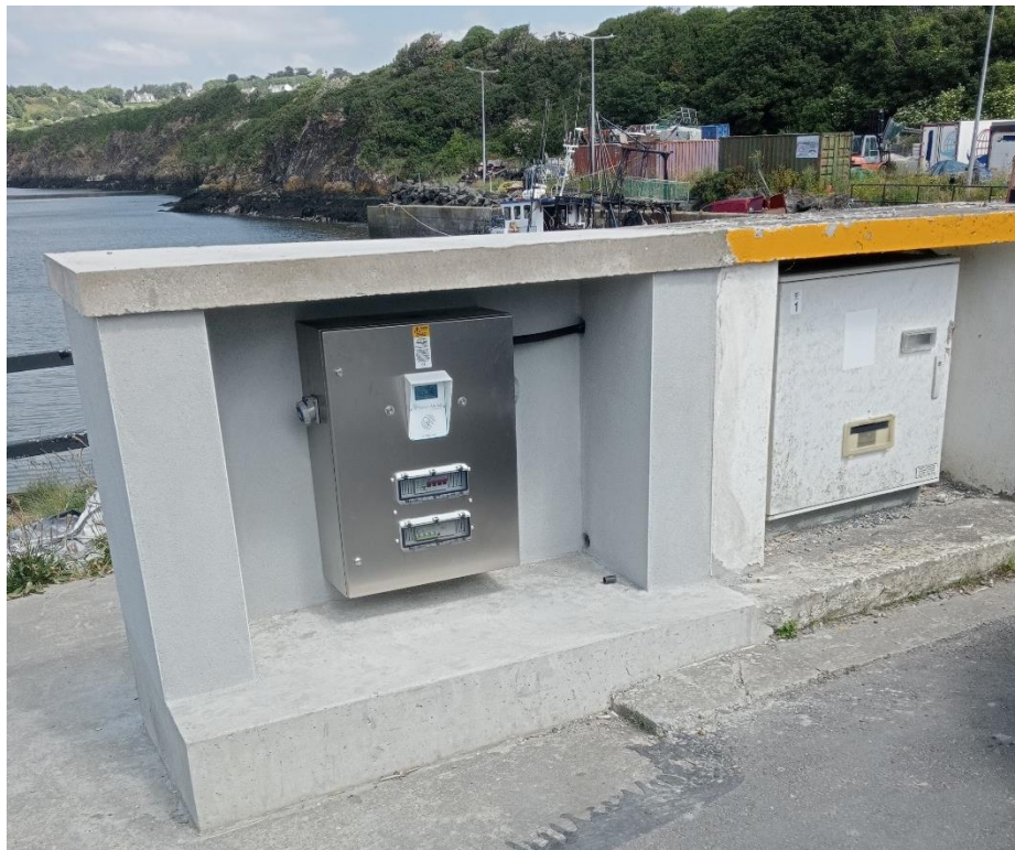
Figure 6-3: Duncannon Harbour Waste Water Pumping Station
