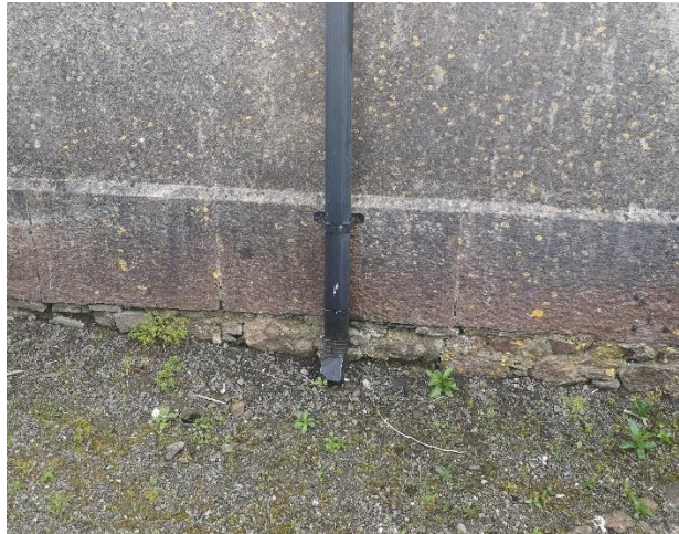
Figure 3-3: Existing Building Rainwater Downpipes (Zone 02)
