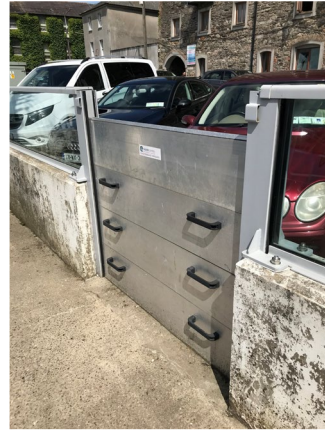
Flood protection blocks access
