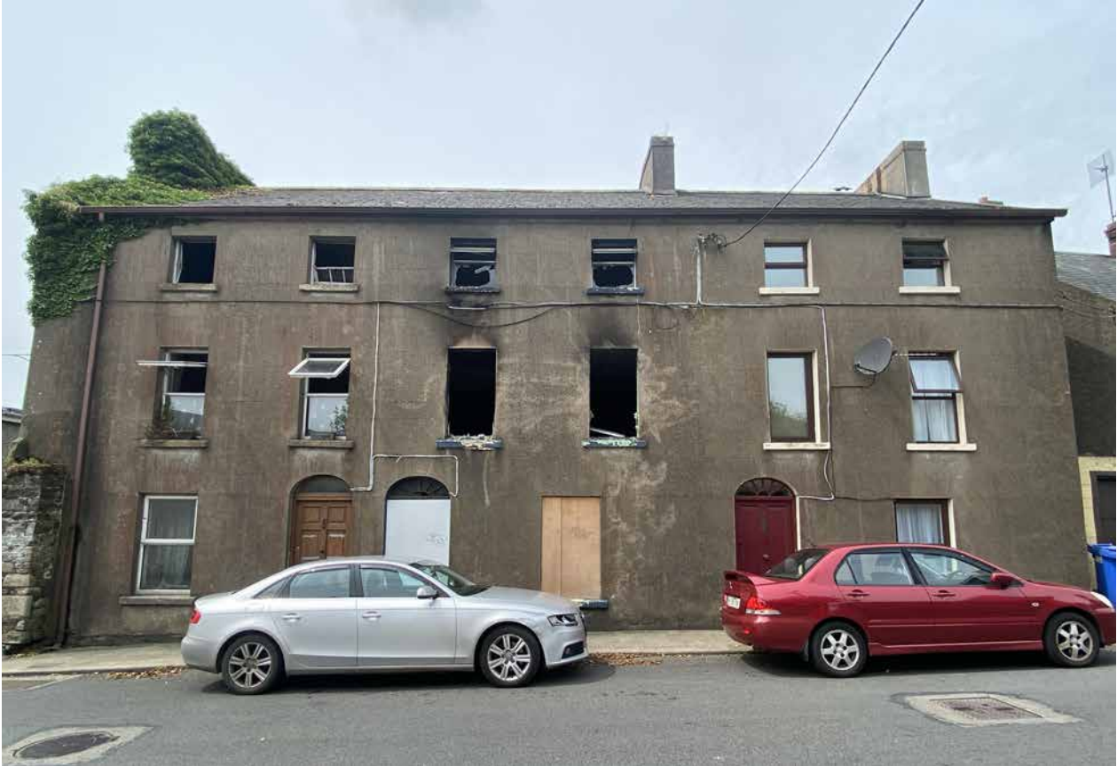
Figure 48 - Burnt out houses
