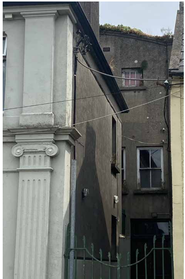
Figure 91 - Poor maintenance evident to structure to rear of YMCA, John Street
