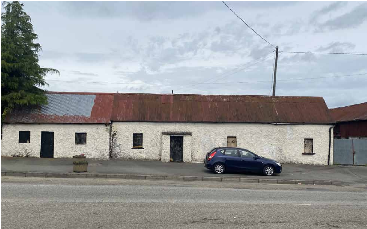
Figure 38 - Vacant historic cottages, Irishtown
