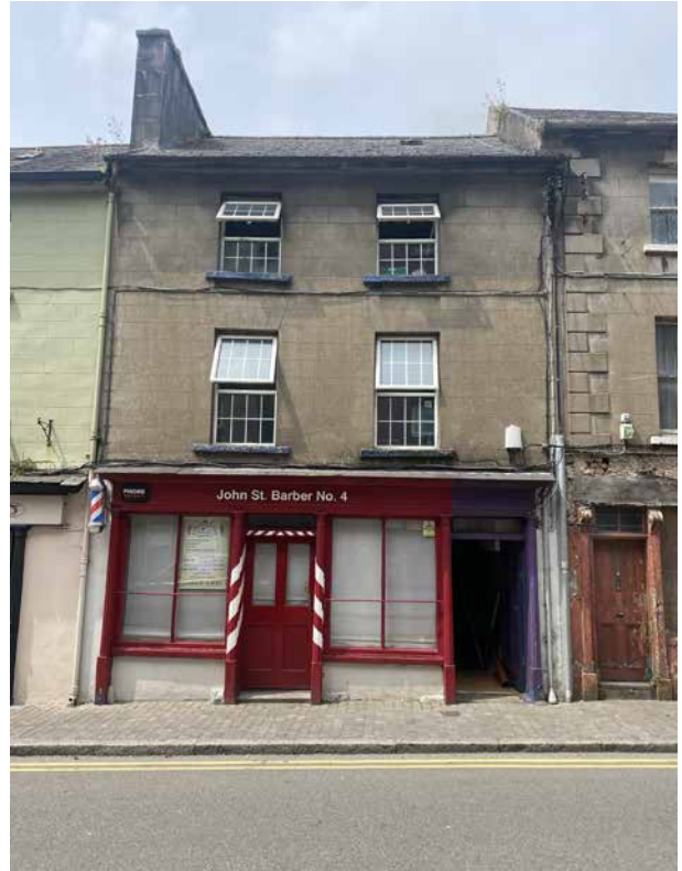
Figure 90 - Inappropriate uPVC windows, John Street
