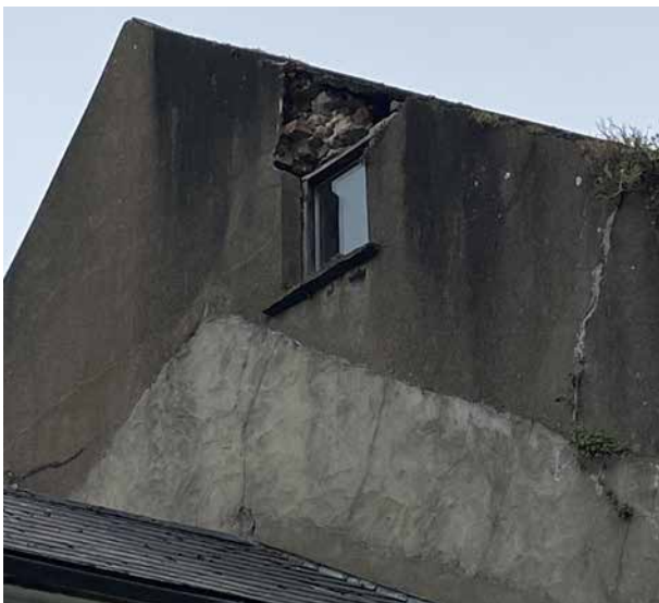
Figure 62 - Poor maintenance, Quay Street
