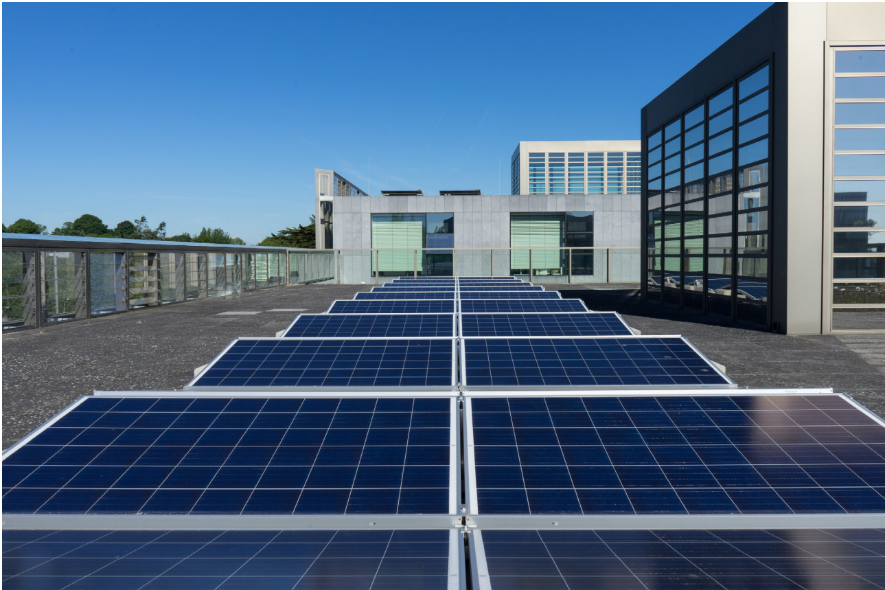
Solar Panels on roof of County Hall Wexford Town (Wexford County Council)
