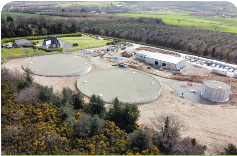
Ballyminaun Water Treatment Plant Investment
