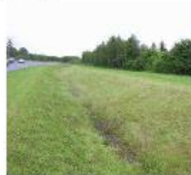
Effectively grassed drains – but wide and mostly dry
