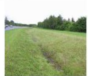
Effectively grassed drains – but wide and mostly dry
