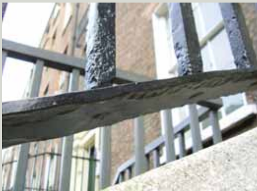
Where new rails are installed, traditional detailing should be matched where possible, such as piercing bars through the rail
