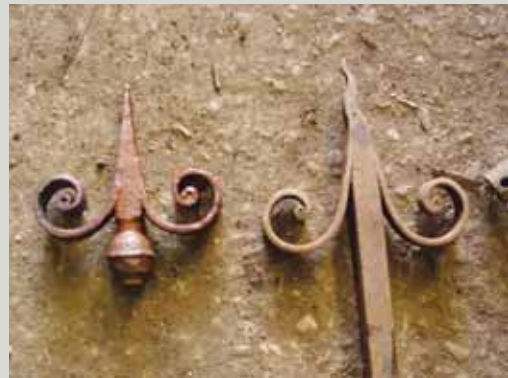
While modern welding techniques are not ideally suited to traditional ironwork, a skilled craftsperson may be able to apply modern welding to repairs to a level that is visually acceptable. The finial on the left has been forge welded and hammered down to a point, while the finial on the right has been electric arc welded and then hammered into a point in the traditional way
