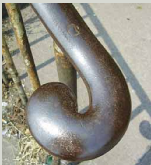
An oxide layer has developed on this wrought iron handrail which protects it from further corrosion
