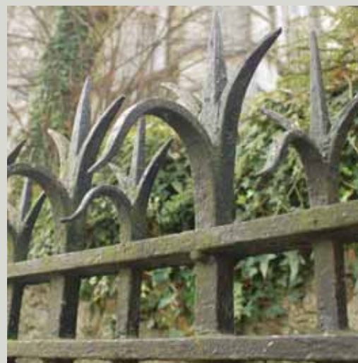
Note the pin just below the top rail of these wrought iron railings which would have been used to hold the rail in place during the assembly of the railings in situ
