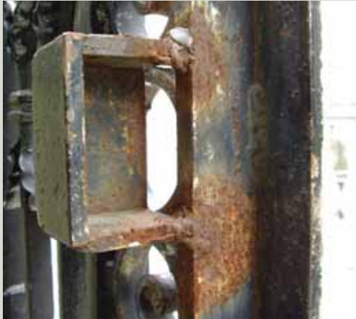
Galvanic corrosion is occurring between the original wrought iron gate frame and the metal of the filler rod that was used to form the weld joint attaching the gate catch to the gate frame
