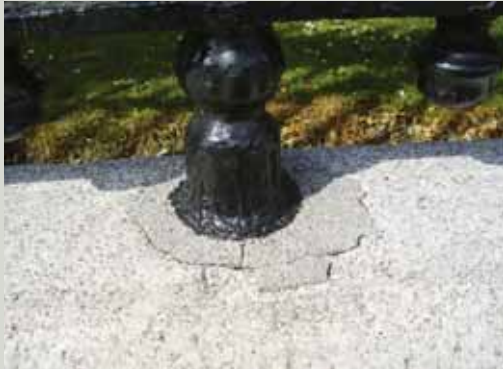
Crushed stone mixed with mortar has been used to fix this ironwork into the masonry socket
