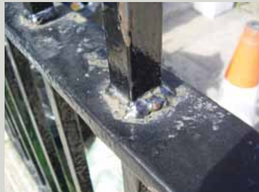
Poorly-finished weld joints can be disfiguring to traditional and new iron and steelwork alike
