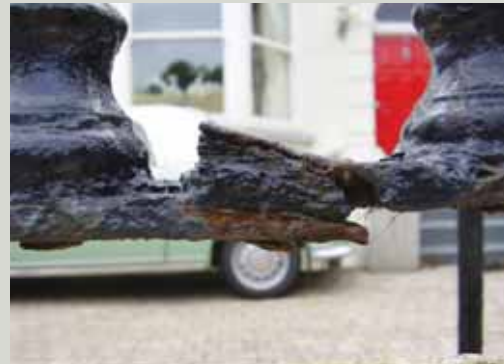
Corrosion developing at a scarf joint
