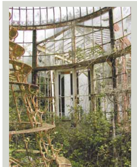
This finely-made circular conservatory was designed and erected at Castlebridge House, County Wexford by James Pierce of Mill Road Iron Works, Wexford. In addition to its iron structure, it contains a 10-tier iron display stand for plants at its centre
