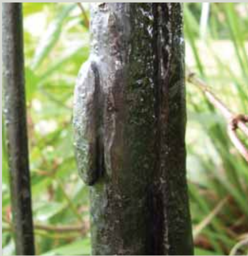
Original wrought iron backstay fixed in place by means of a bradded (riveted) pin
