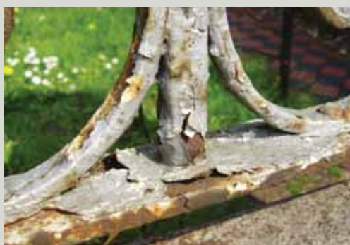
Broken, flaking paint traps and holds water to the iron, preventing it from drying out properly, and can lead to corrosion. Areas of chipped paint are not as significant a threat so long as the iron is in an exposed location and is able to dry out. Nevertheless, such chips should be treated as soon as possible to prevent rust from forming
