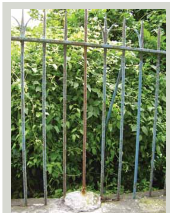
Repairs should be sympathetic to the design and traditional detailing of ironwork unlike this repair which is damaging to the appearance of the railings, will damage the stone coping and is likely to fail
