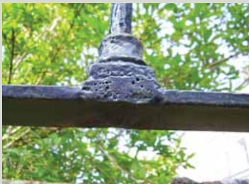
Paint cannot fill holes. Casting flaws such as those pictured above should be filled to prevent water becoming trapped and causing corrosion to develop
