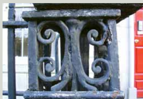
Posts from two different properties on Parnell Square, Dublin. While appearing to be severely corroded, much of the original ironwork in the lower example may remain intact beneath layers of paint and corrosion
