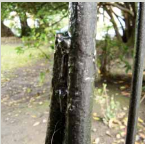
This backstay has been repaired by welding it back into position, which is not in keeping with the traditional techniques used to assemble this railing
