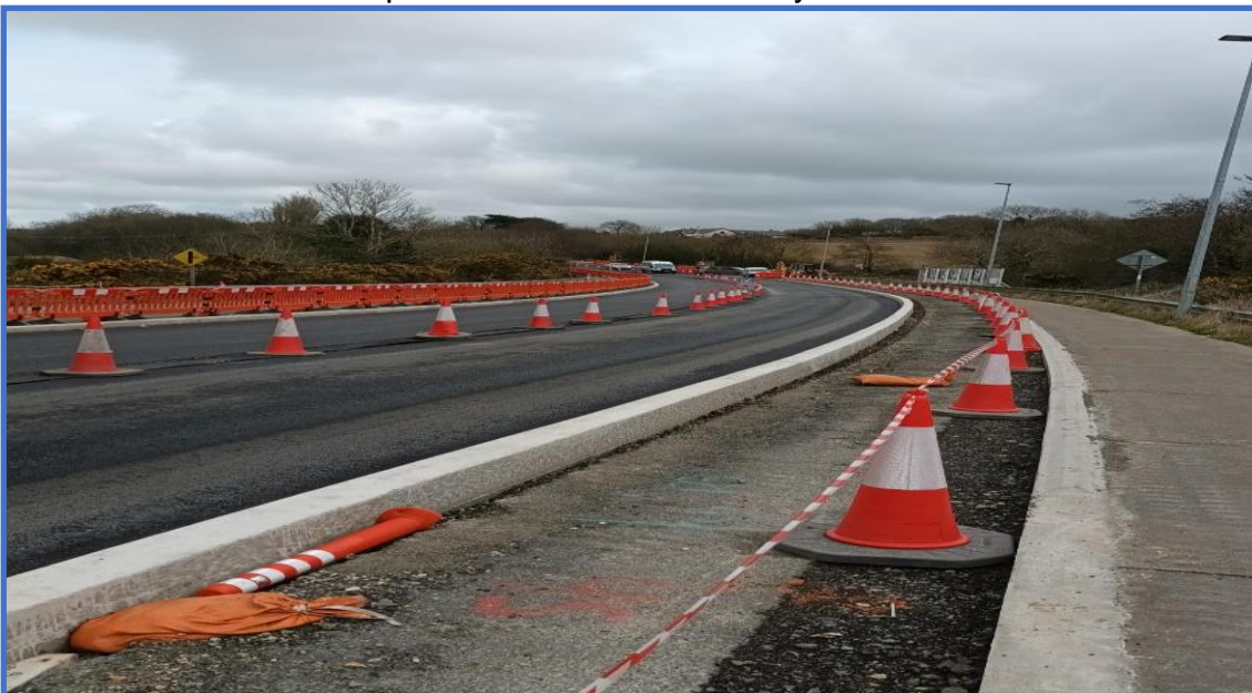
Slip form kerbing to edge of new protected cycle path at Newtown Road
