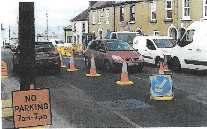
Image 11 Roadworks on William Street Lower during the traffic survey between Thursday, 5th to Thursday, 12th September
