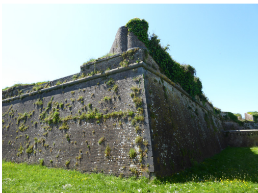
Fig. 106: Battered walls north of bridge entrance
