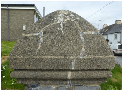
Fig. 134: Extensive cracking to pier cap
