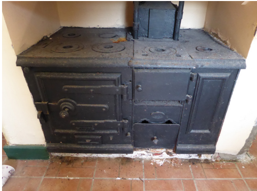
Fig. 57: Range in kitchen area
