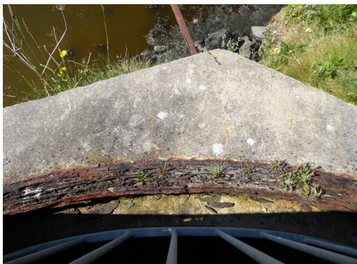
Fig. 12: Corroded iron tracks to screens
