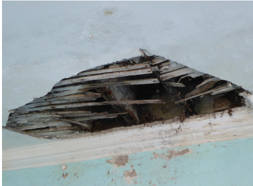
Fig. 58: Collapsed plaster to lath and plaster ceiling
