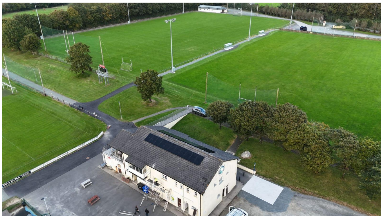
Solar PV installed at Glynn Barntown GAA Club funded through CCAP
